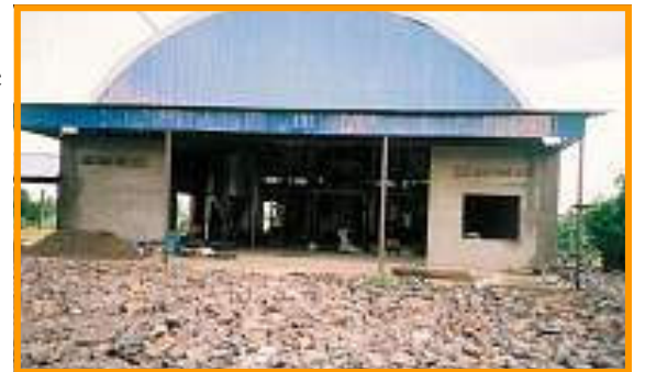
Rice mill — large rock had to be brought in to keep the 20 ton loads coming out of the mill from sinking.
